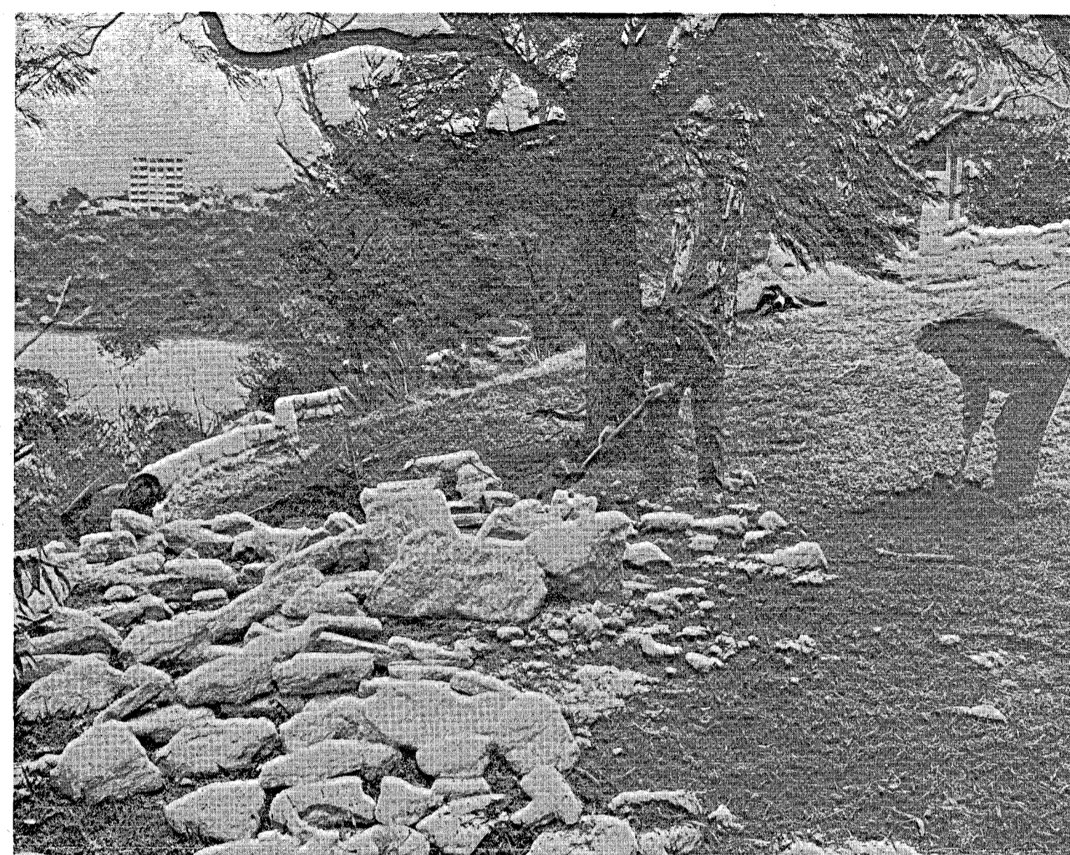
Here, three members of the ground staff work on the landscaping of the river bank, the edge of which is marked by the limestone wall. The Chapel can be seen in the right background.
