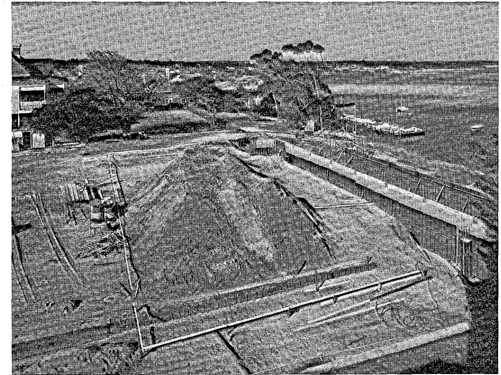
The Chapel site, taken from Queenslea balcony looking east to "Romsey" on left and "McClemans" in background. Tyre marks run across future courtyard.
